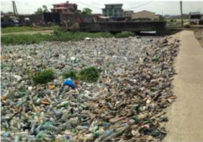
Plate 1. A Section of canal at Orefero Street, Shomolu LGA of Lagos state, filled with municipal solid waste of all descriptions Source: Authors' Field Survey, 2014.
