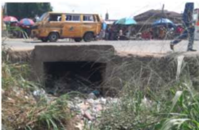
Plate 5. Drainage intersection blocked with MSW along Agege Motor Road, Agege Local Government Area of Lagos State, Nigeria Source: Authors' Field Survey, 2014.
