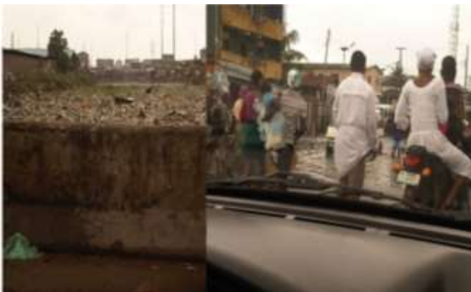
Plate 7. Solid waste blocked drainage channels and caused flooding along Bakare-Faro Street, Ajeromi-Ifelodun LGA, Lagos, Nigeria (Source: Authors’ Field Survey, 2014).
